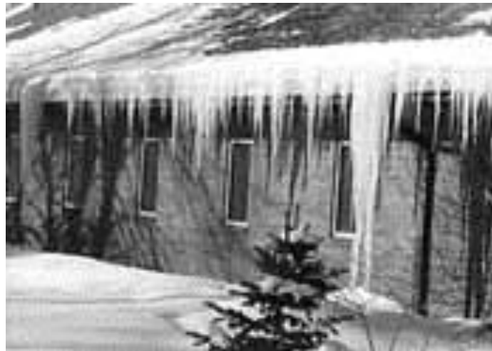
This wintry scene is brought to you by high heat loss. The ice dam at the roof's edge is damage waiting to happen.
