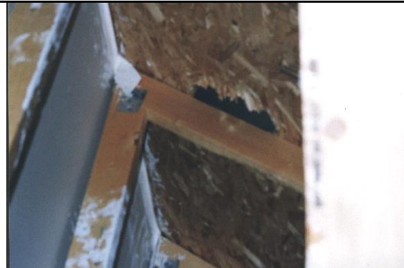
Photo 4 - Typical opening made in OBS (strand board) for roof vent (Note: jagged edges)
