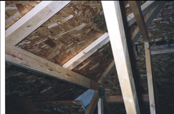
Photo 1 - Typically 2 x 4 rafters installed on the flat instead of edge
