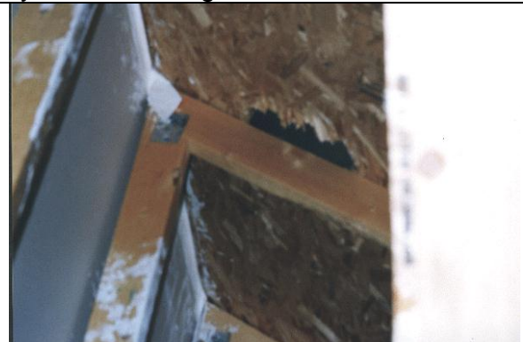
Photo 4 - Typical opening made in OBS (strand board) for roof vent (Note: jagged
